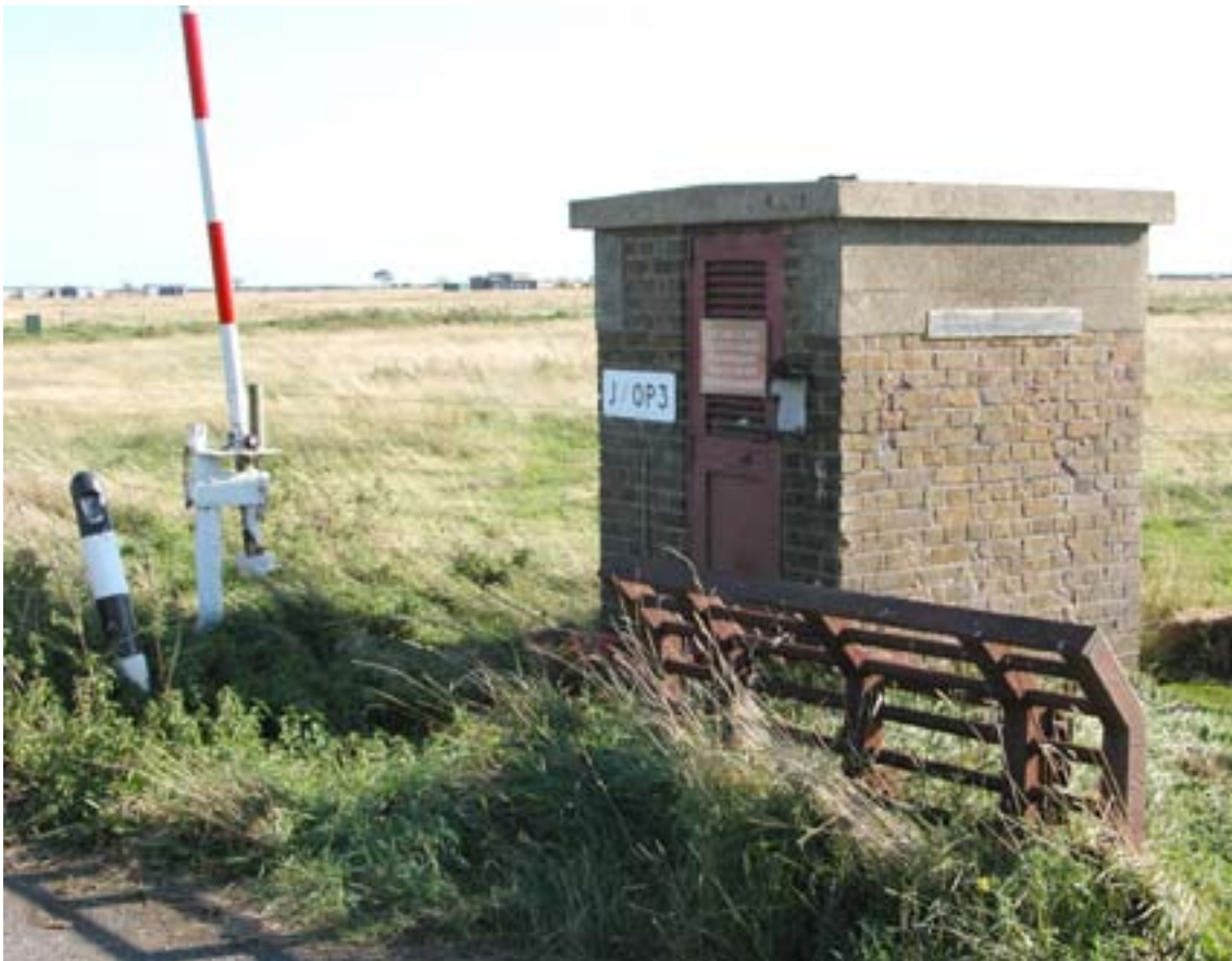
Figure 19: J/OP3 this brick Observation Post with narrow observation slits is typical of such posts built in the late 1940s and early 1950s. (c) English Heritage
